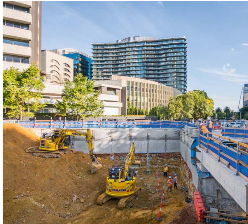
↓ Construction of Anzac Station, located in a residential quarter; required adjusting working hours and communicating regularly with residents.
