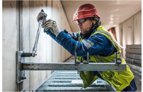
Fernando Cardoso, an employee of a partner company, installs cable duct supports in the underground tunnels.
