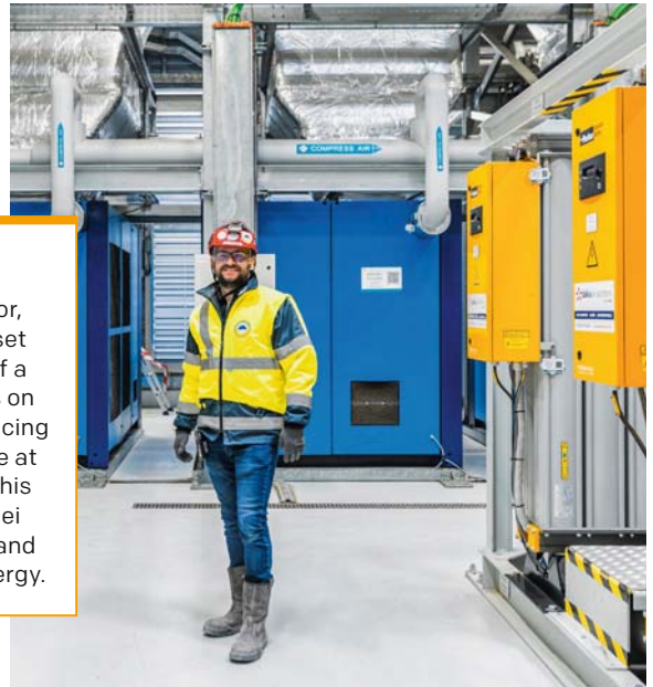
↓ Anthony Guilbert, an Equans project leader, in the Equans-designed plant for the production of demineralized water, compressed air for certain types of equipment like valves, and air for oxygen masks.
