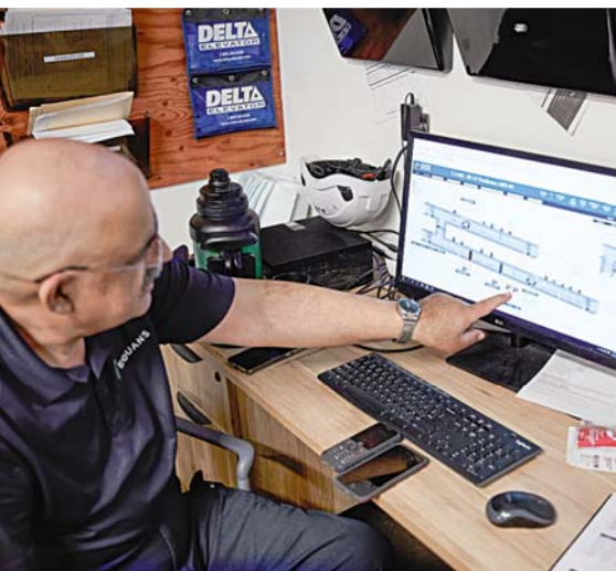
← ↓ Technicians monitor the hospital's energy consumption using a building automation system.
