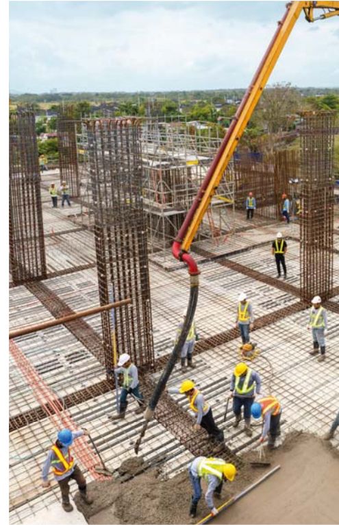
↓ Some 2,300 construction workers are on the job night and day, seven days a week at the data center site.
