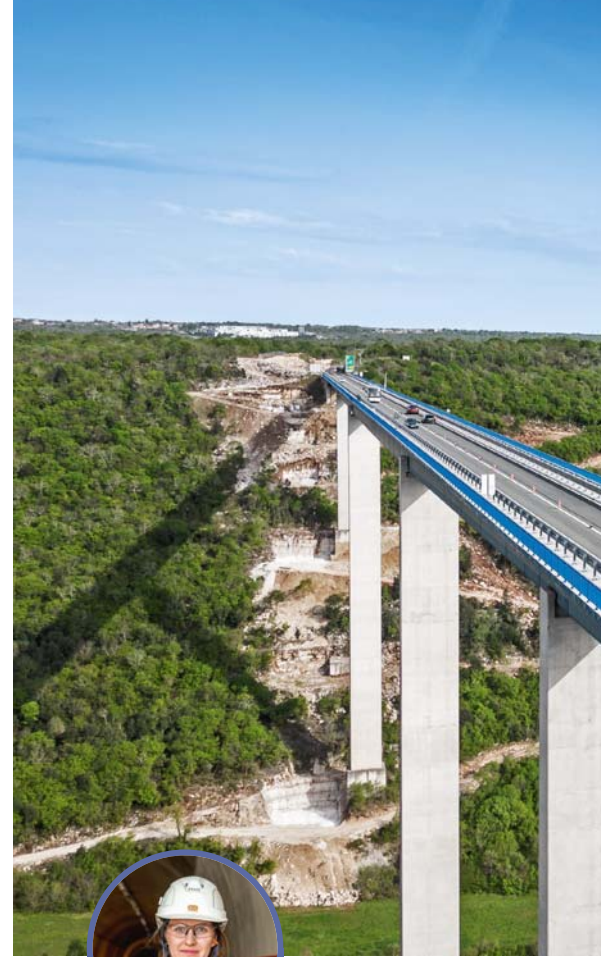
→ The Limska Draga Bridge, with its 110-m piers, will soon be twice as wide.
