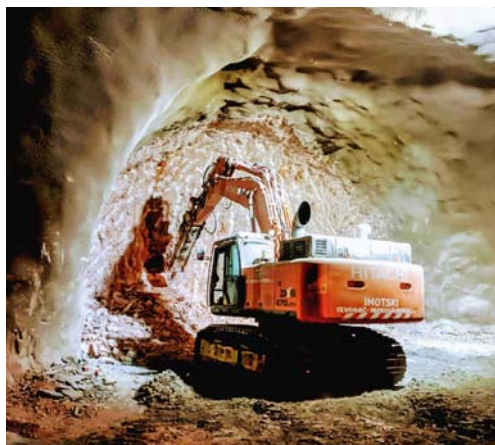
↓ A Jumbo does the drilling in the excavation of the Učka tunnel.
