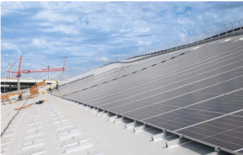
↓ The 4,680 sq. m of photovoltaic panels will supply 25 percent of the facility's electricity consumption.
